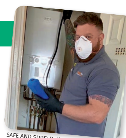
SAFE AND SURE: Boiler Plan engineers arrive at MMHS properties in PPE gear.
